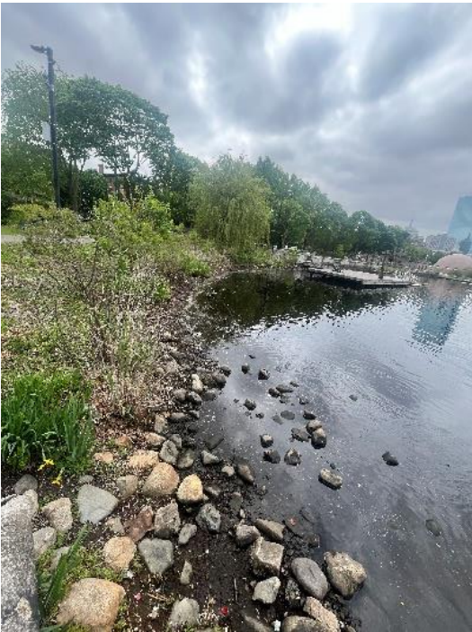
Deteriorated riprap shoreline.
