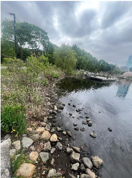
Deteriorated riprap shoreline.
